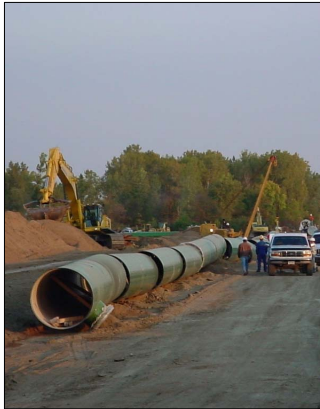
Construction of a MR&I Water Supply Project Similar to the Proposed Project
